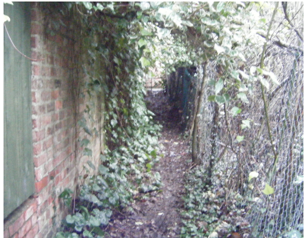
Photo 4 Narrow and overgrown section
